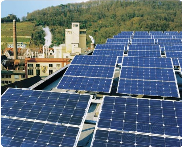
Brauerei Ganter (brewery), 70 kWp, Freiburg i. Br., Germany
